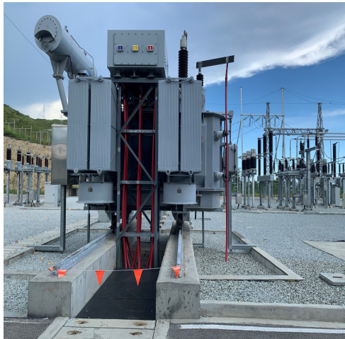
Kilakila substation in Badili district
